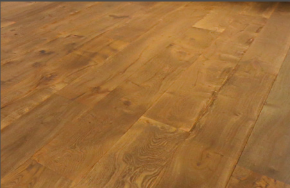
ENGINEERED TIMBER FLOORS W/ SATIN WAX FINISH
